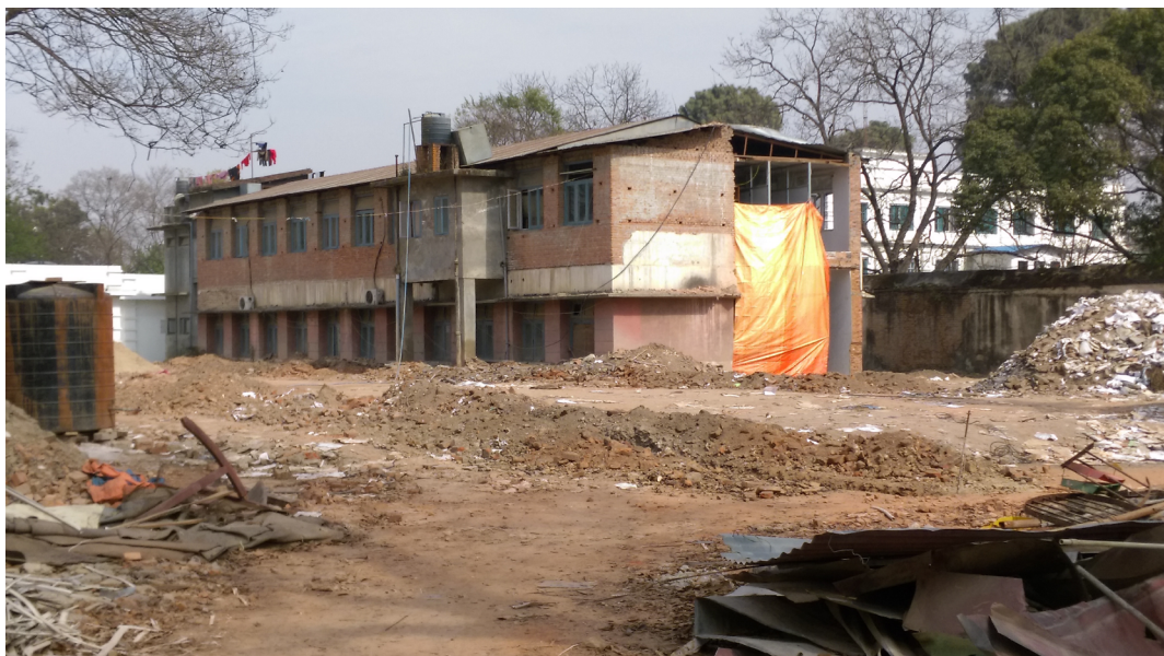
An earthquake-damaged government office building in Singhdurbar, Kathmandu on February 3, 2017. Photo Credit: Prachi Agarwal for JustJobs Network
